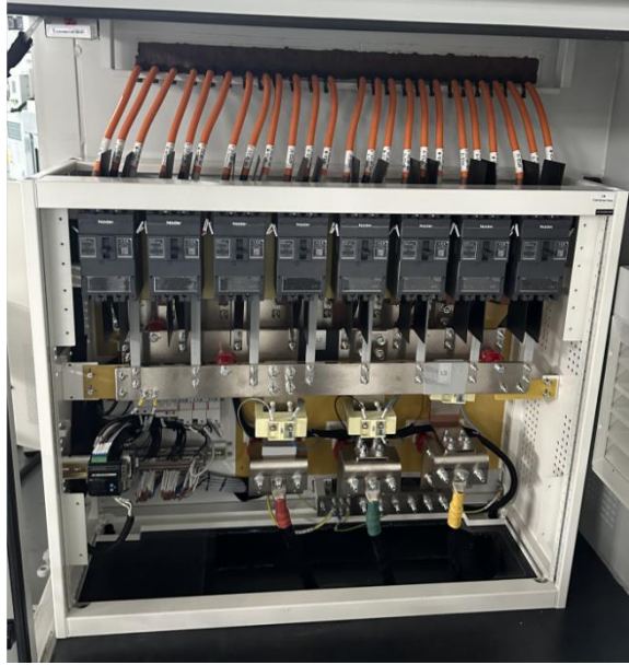
Figure 6-4 The door of primary distribution box opened
